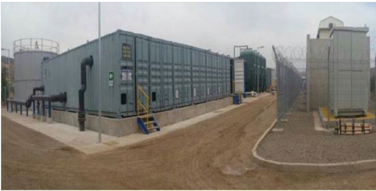
View of the nanofiltration containers at the plant.
