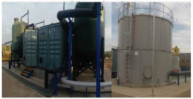
Sand filters and runoff tank.
